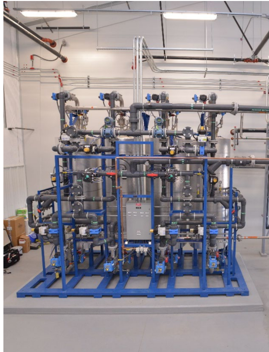
IX resin vessel skid
