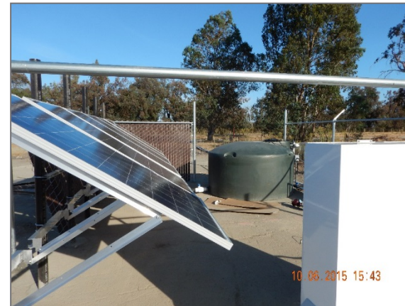
Upland Irrigation Station Setup
