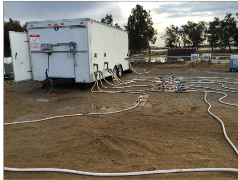
Injection Trailer and Manifold
