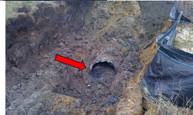
Culvert with fuel contamination
