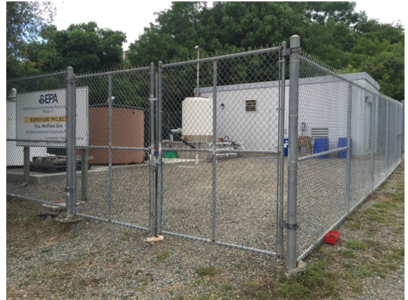
Remedial system components
