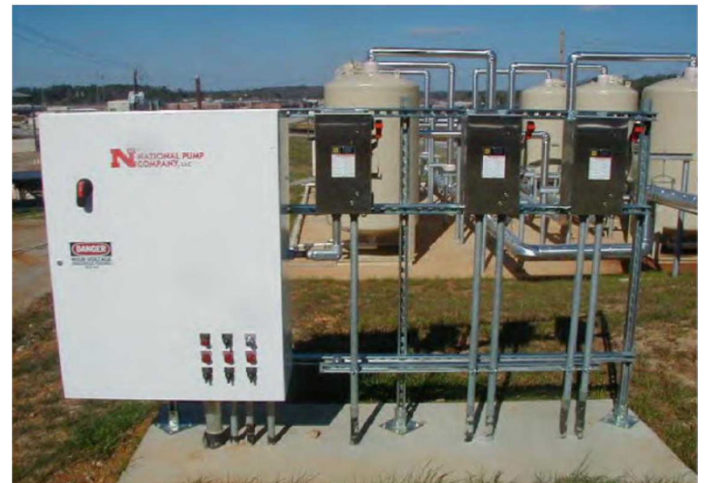
Electronic pump control panel
