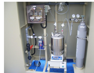
Culture injection unit by using N 2 cylinder
