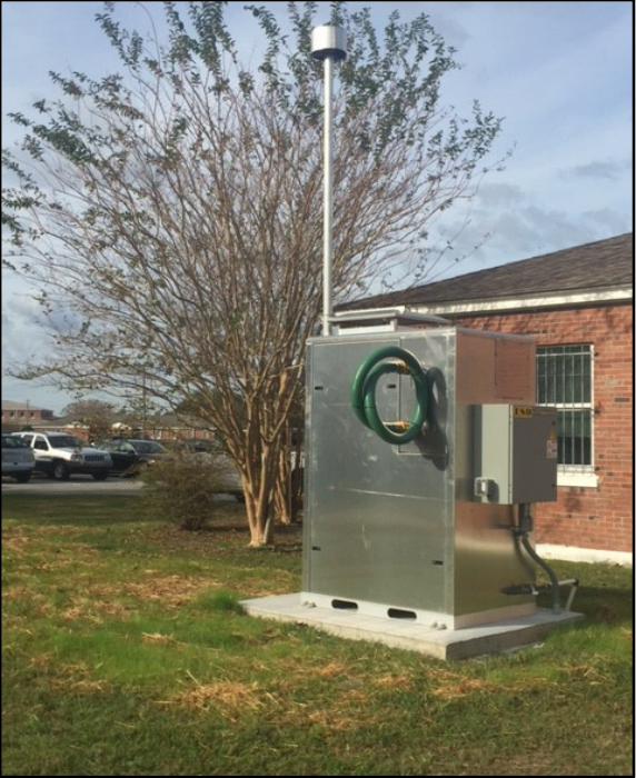
Blower Enclosure and Stack
