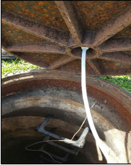
Manhole Sample Port
