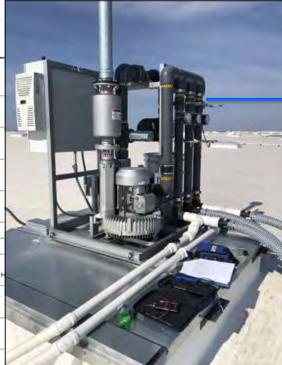
6 blower skids (roof)
