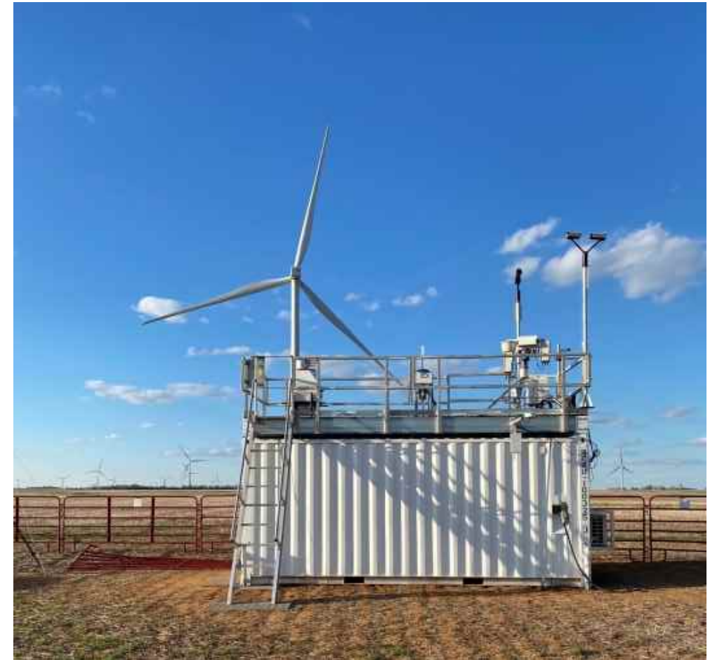
Instruments installed at site A1. Photo from Raghavendra Krishnamurthy
