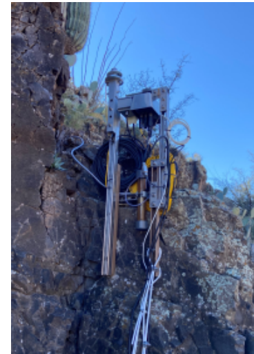
Sycamore Creek (SYCA) in AZ: Solar Power
