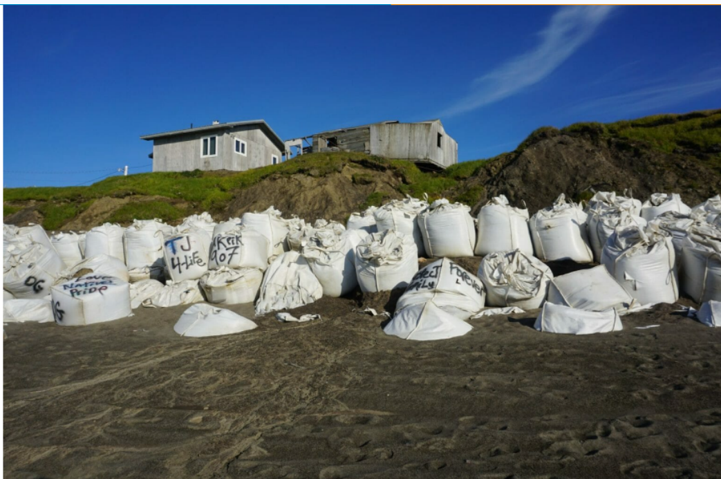
Houses, seen on Aug. 2, teeter on the edge of an Utqiagvik bluff that is being rapidly eroded by permafrost thaw. The house on the right has been abandoned. At the base of the bluff are SuperSacks filled with sand, placed there as part of the effort to hold back ocean waves and slow down erosion. (Photo by Yereth Rosen/Alaska Beacon)
